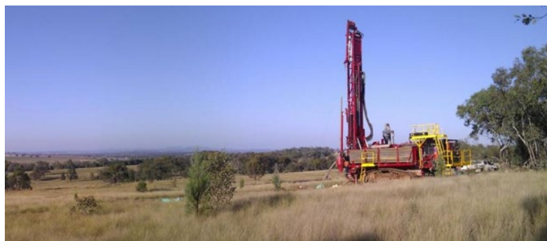
Reverse circulation (RC) drilling may also be undertaken using a larger rig.
